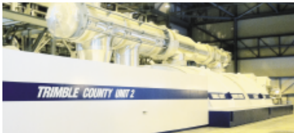
The Trimble County 2 turbine.
